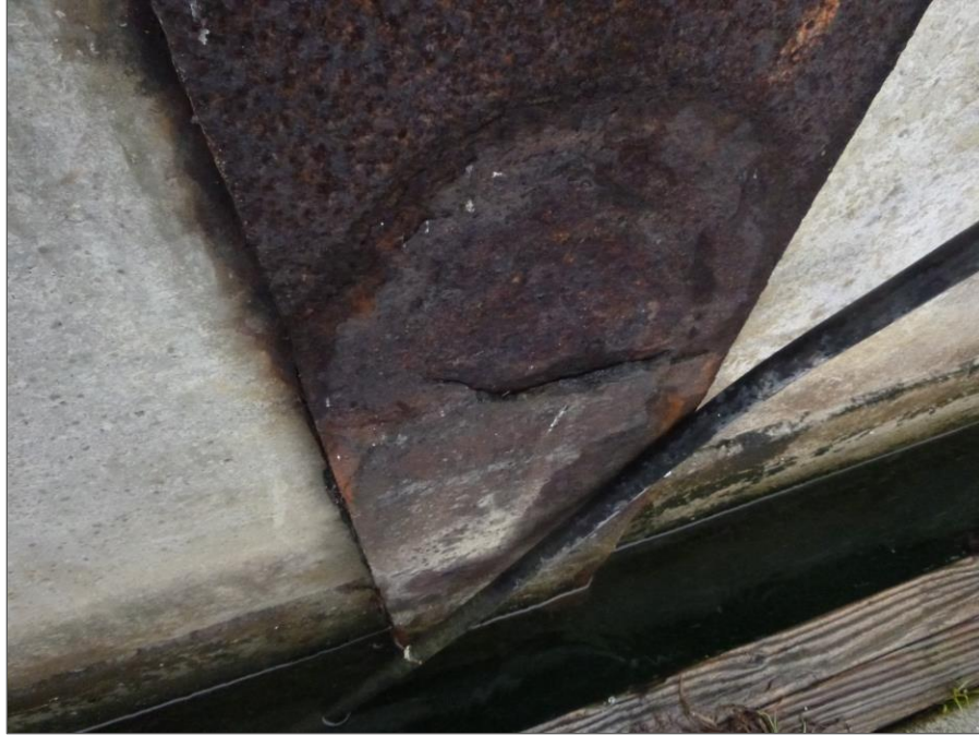
1(c). Typical chloride-induced corrosion damage in splash zone (8 October 2018)
