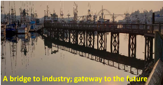
Holes in the existing pilings
