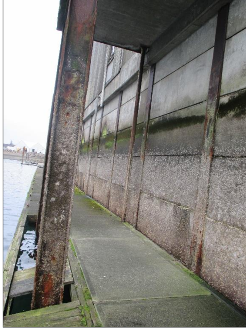
Figure 2. Concrete lagging existing conditions (There are surface effects from water; however, the overall visual inspection seemed acceptable at this point.)
