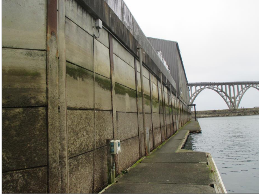
1(a). Corrosion on soldier piles (27 February 2018)
