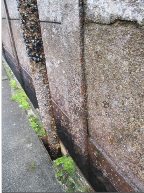
1(e). Formation of calcium carbonate shows the possibility of carbon-induced corrosion (27 February 2018)
