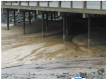
(Figure 2) Sediment discharged into the marina in February, 2016 from Outfall #1
