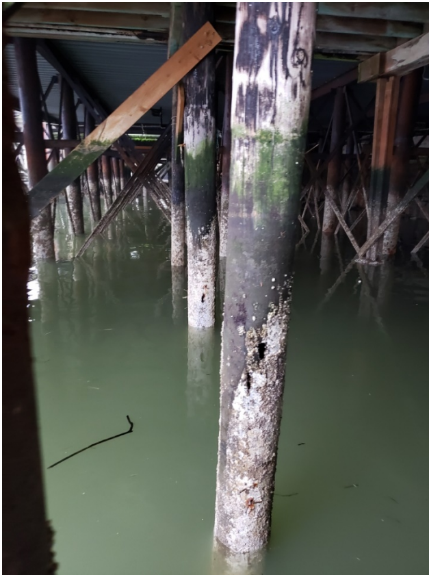
Figure 3 Holes in the pilings in the foreground and background. Foreground piling is out of vertical, not supporting full load
