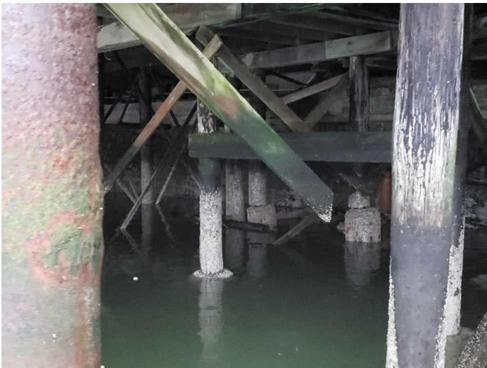
Figure 4 Pilings in the background have shifted on their bases to the left, and the bases are leaning due to undermining
