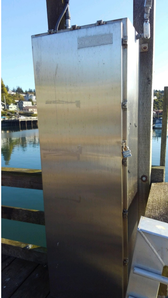
Figure 1 Port Dock 5 Breaker Cabinet
