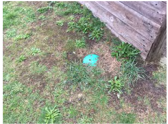
Picture #29. Utility access
